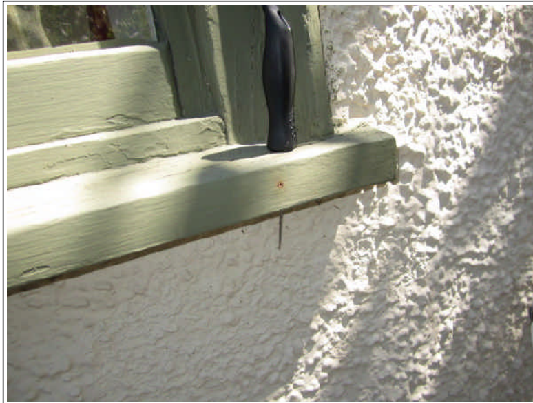
Action Necessary - There is sections of rot in some window frames.
