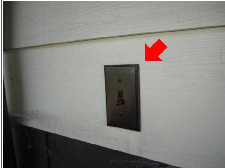
Attention Needed - an internal light switch has been used externally.
