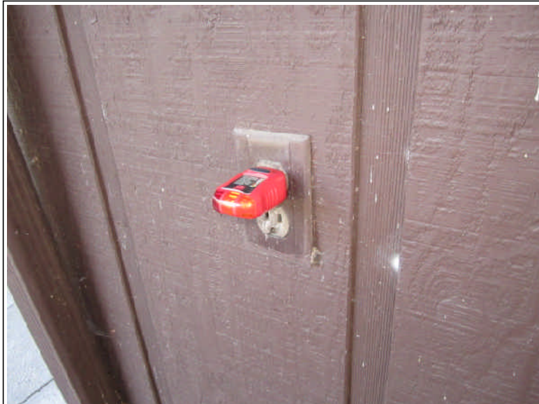
Action Necessary - The external outlets are not GFCI protected. This type of protection should be installed on all external sockets.
