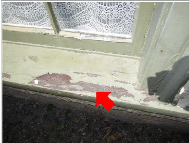
Attention Necessary - Some exposed wooden surfaces are in need of painting/staining.
