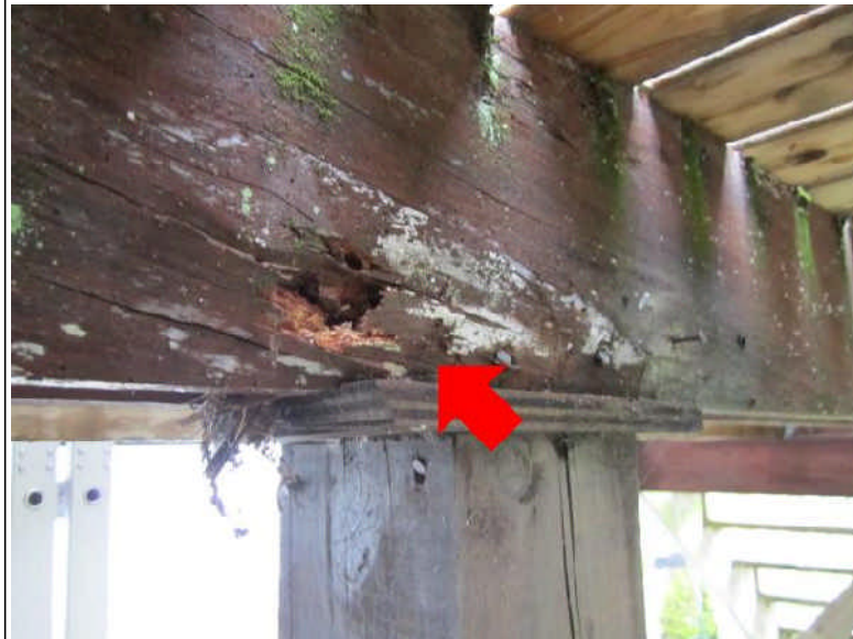
Action Necessary - Sections of the beam(s) are rotten.
