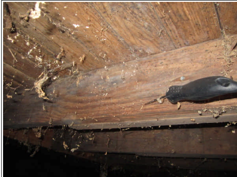
Action Necessary - Sections of the joists are rotten.
