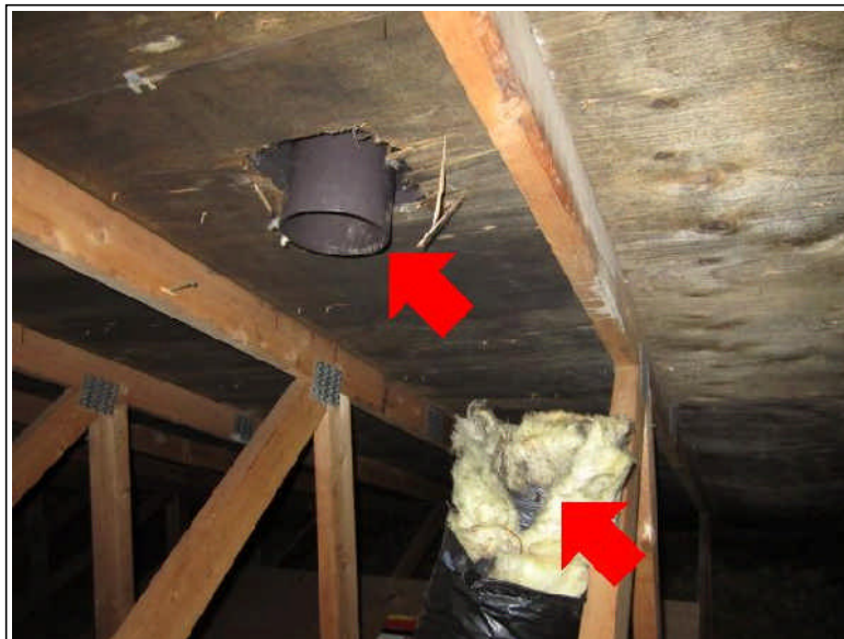
Action Necessary - A dryer vent is discharging into the attic space. Mould has formed on the underside of the roof sheathing. It is strongly recommended that the services of an environmental consultant are used.
