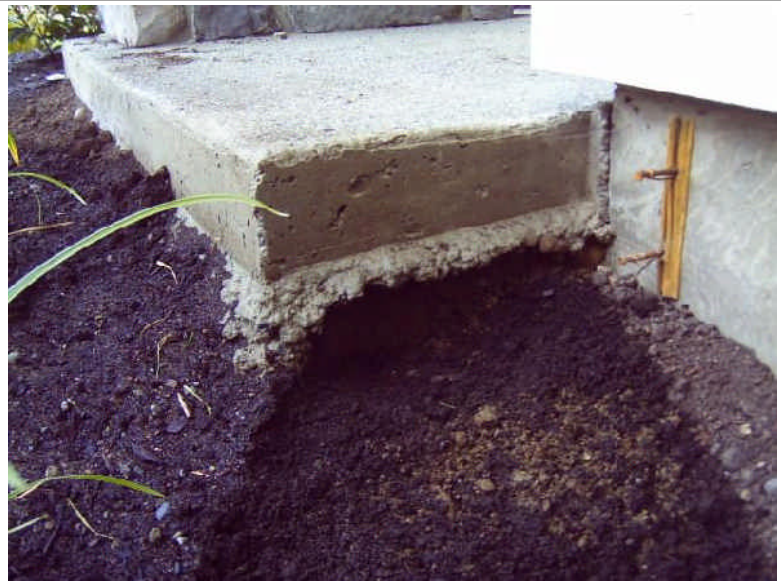
Action Necessary - The edges of the concrete porch floor are inadequately supported. This will eventually cause the concrete to crack.
