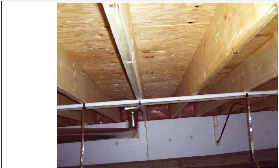
Attention Necessary - some of the larger joists spans didn't have any cross bracing.
