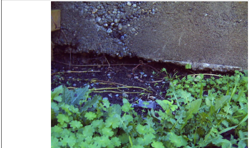
Attention Needed - The retaining wall at the rear is poorly supported, there are gaps underneath. The one on the right is satisfactory.
