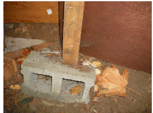
Action Necessary - the columns are poorly supported.
