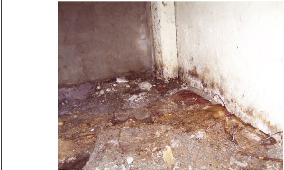
Action Necessary - there are rotting columns, access door and wall under the stairs.
