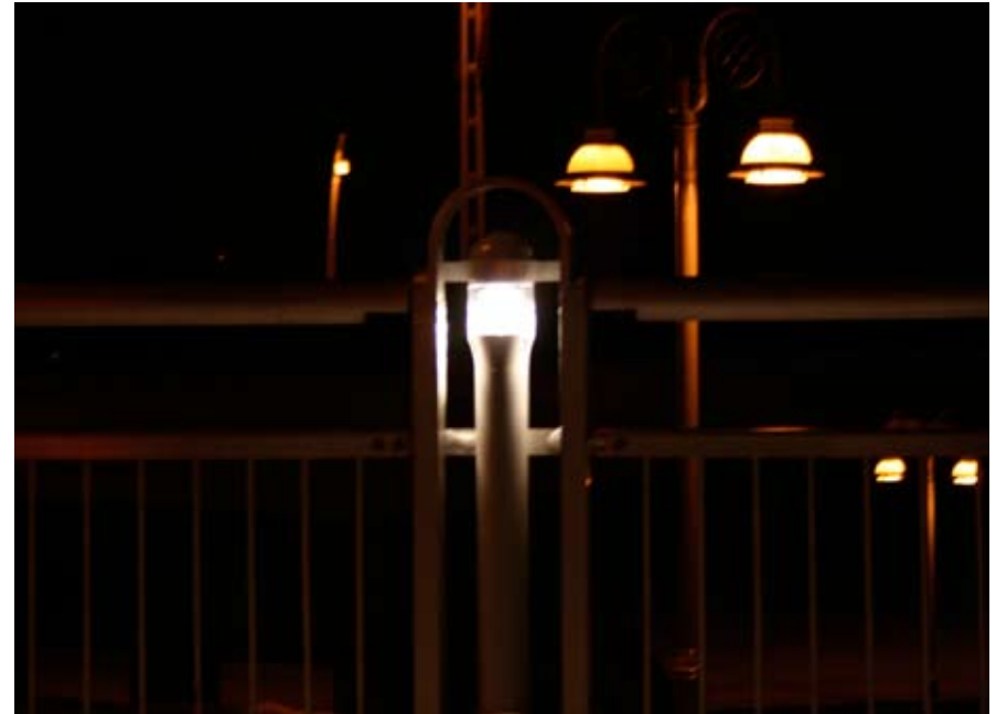
Post mounted railing lights.
