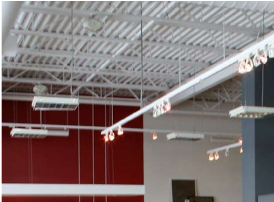
Fluorescent diffuse downlights.
