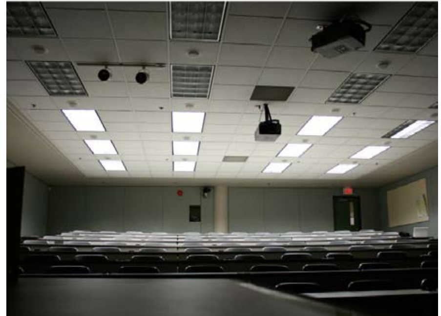
Controllable banks of fluorescent fixtures.
